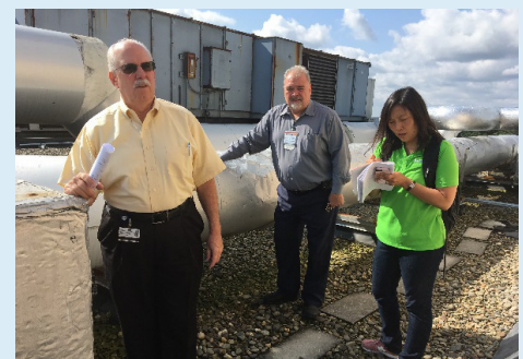
Abington Health Center-Warminster Charles McClinton, Supervisor, Randy Haines, Director of Energy Management, Damee Choi, AECOM
