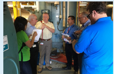
Jefferson Torresdale Hospital Damee Choi, AECOM, Randy Haines, Director of Energy Management, Jim Creighton, AECOM, Jim Zernhelt, Project Manager, Alex Martinez, Martinez CX, Kevin Whitten, AECOM
