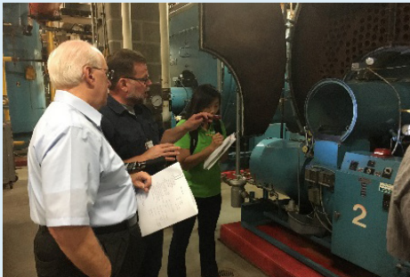
Jefferson Bucks Hospital Randy Haines, Director of Energy Management, Keith Jellyman, Supervisor, Damee Choi, AECOM
