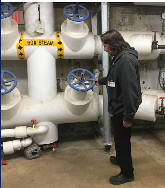
Frank Mirarchi, Facilities Services Supervisor, checks steam equipment in Jeff Hall.
